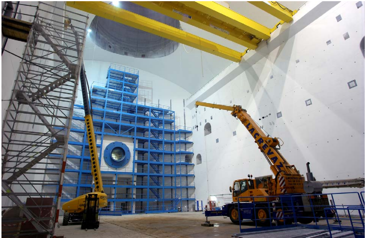
Figure 10.2: The UX15 cavern for the ATLAS experiment shortly after reception by CERN from the civil engineering contractor
