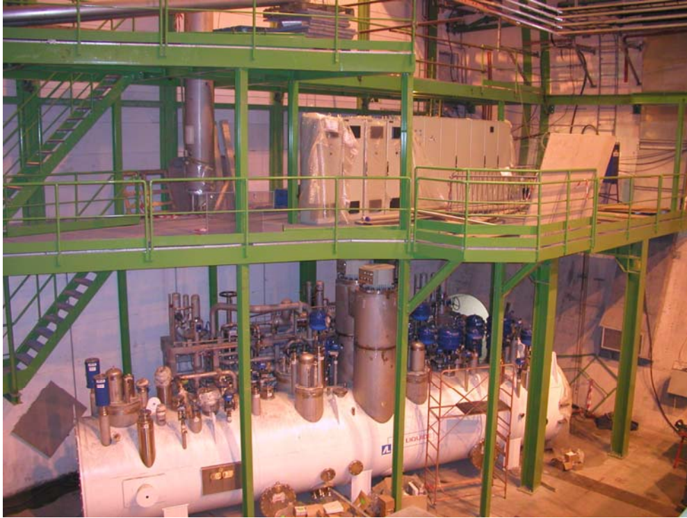
Figure 10.12: Picture of the QUI interconnection box in its final position
