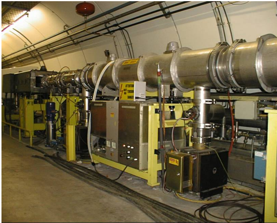
Figure 14.1: The SPS damper H1 (BDH214.37) with its power amplifier installed below the kicker tank.
